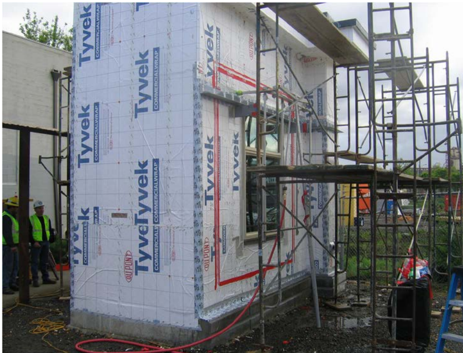
Figure 9. Exterior wall assembly mockup, including air barrier materials and components. Mockup shown under negative pressurization during quality assurance testing.
