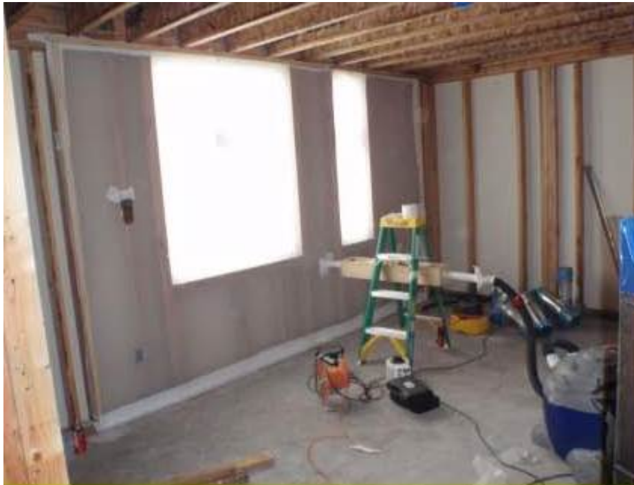
Figure 10. Air barrier assembly testing in progress. (Photo courtesy of RDH Building Sciences)
