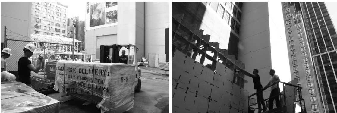
Figure 13 first of 10 bundles of plywood cut in Virginia and assembly of contouring structure from the wall to the roof
