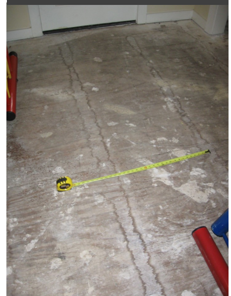
Figure 2. Subfloor with moisture damage in a house with impermeable vinyl flooring (removed) above a vented crawl space
