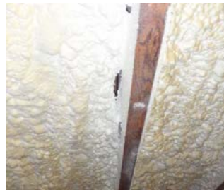
Figure 3: Delamination at rafters
