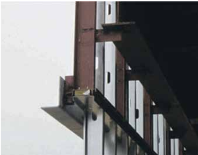
Figure 9. Stand-off. This can be welded to plates cast into slabs or welded to structural.
