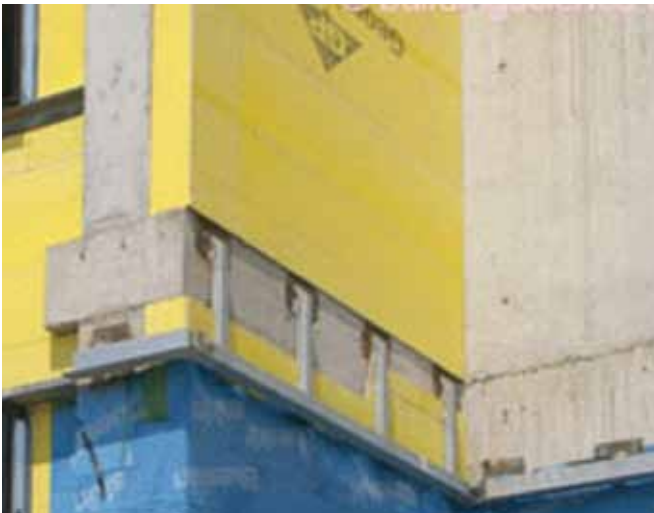
Figure 10. Relieving angle line up. Notice how the relieving angle lines up with the top of the window.
